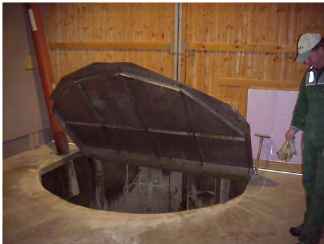
Photograph 6.3: Underground mixing tank of Biogas plant Paldau
