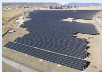
2 MW PV system at U.S. Army Fort Carson, NREL Photographic Information exchange
